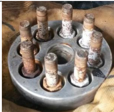
LOOSE OR DAMAGED FITTINGS
